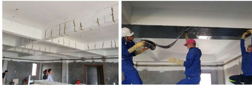
Fig 1. Cracked and deflected RC beam strengthened by CFRP
