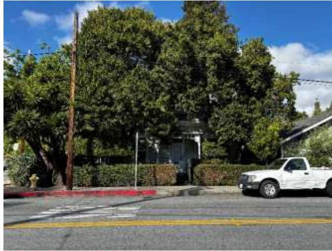
Figure 3. Example Extreme-Risk home (Neighborhood 1). Visible features include combustible wood siding, single-pane windows with wood frames, limited defensible space, and vegetation/branches in contact with the structure.
